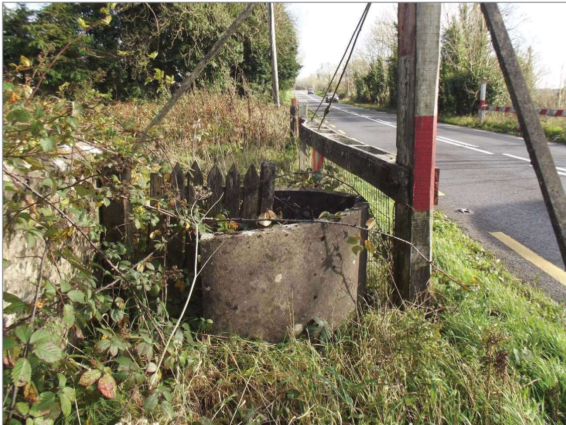
Illus. 5.7 and 5.8—Railway crossing on the N17 (Inventory No. 7). Options 1 and 2 would affect the boundary wall and pedestrian stile (below); Option 2A would result in the demolition of the keeper's cottage also, which is rated a severe impact of the road project.
